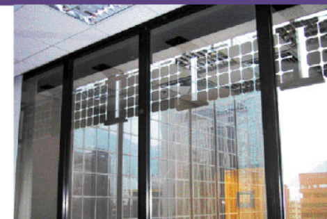
灣仔政府大樓的光伏系統 PV system at Wanchai Tower
