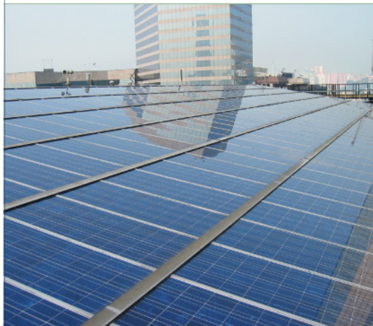
灣仔政府大樓天台的光伏板。 Photovoltaic panels on the roof of Wanchai Tower.
