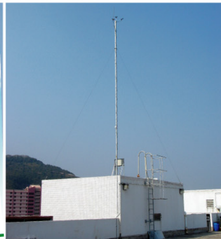
首個風力監測站設於政府物料營運中心的天台。 The first wind monitoring station was set up on the roof of the Government Logistics Centre.
