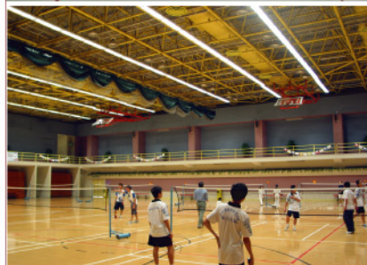
用數碼定位照明界面系統控制 T5 管 T5 tubes controlled by DALI system
